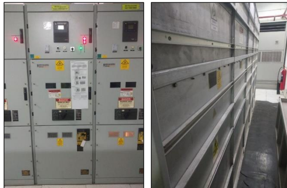
Gambar 2. Kondisi MV Switcgear Didalam Cement Mill Substation
