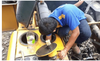
Gambar 5 Flushing Hydraulic Tank
